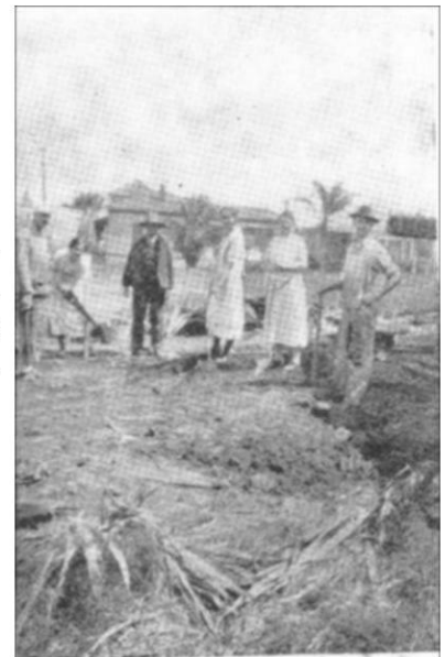
Digging the foundation of the new Mexican church Mr and Mrs Thomas will be seen on the right
