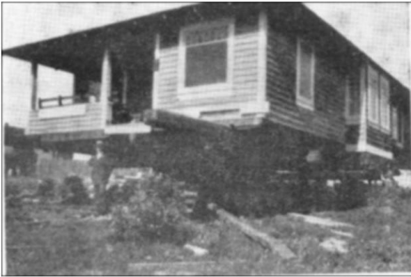
The new home being lifted off the foundations, and moved further back to make room for the new church
