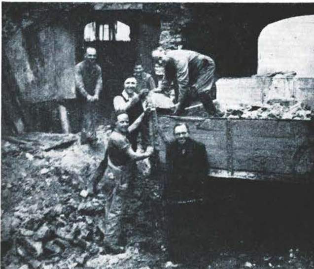
Clearing out the rubbish in preparation for the building of the new Elim Church at Plymouth. Pastor J. Kennedy joins with his members in a labouring job as the preliminary to greater things to come. We shall look forward to news of the completion of this plan.
